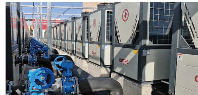
Liaoning Province Dalin City Vocational Technical School Heating Area: 150,000m 2 Heat Pump: mixed models Total: 130Units
