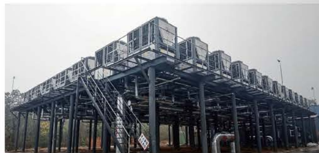
Baizhai Town, Xinmi City, Henan Province Heating Area: 600,000m 2 Heat Pump: 150kW/unit Total: 130Units
