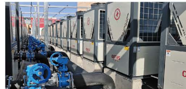
Liaoning Province Dalin City Vocational Technical School Heating Area: 150,000m 2 Heat Pump: mixed models Total: 130Units
